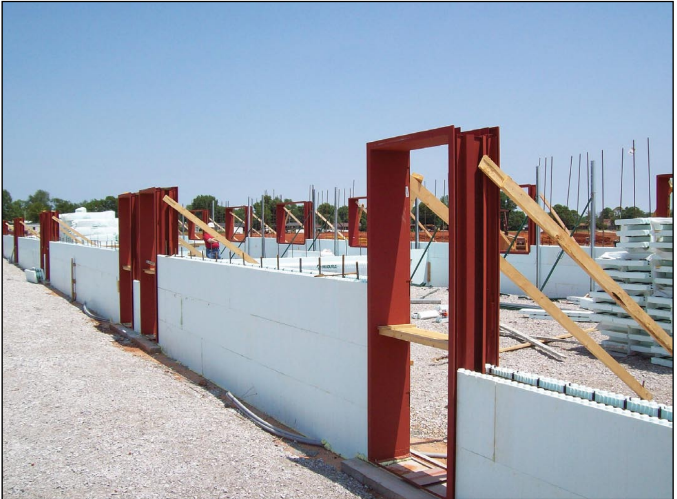
▲ IFA doors installed prior to concrete pour at Joseph Warren Middle and High School (Bowling Green, KY). Note IFA windows in background.
