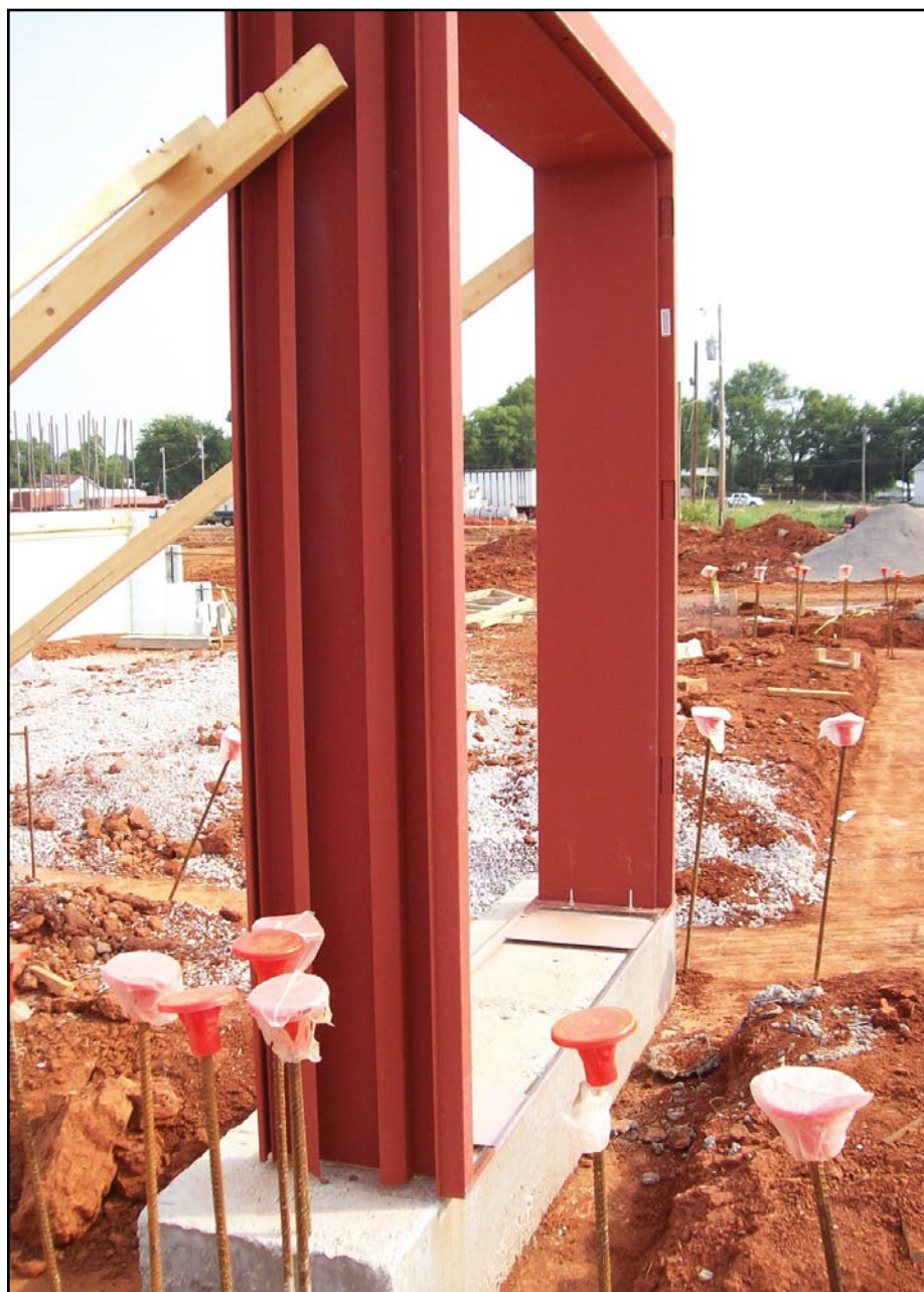
(Joseph Warren High School/Middle School, Bowling Green, KY, photo by Stala Integrated Assemblies, LLC).
