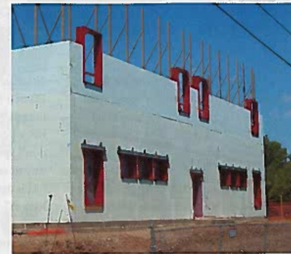
Shown here are the first and second floors of ICF block, stacked around door and window IFAs. This method was used with all 300 of the Academy's openings.
