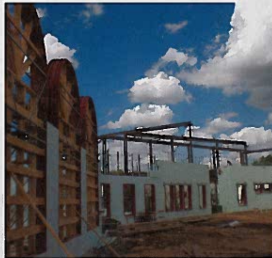
The Academy's unfinished interior. ICF block is stacked around door and window IFAs.
